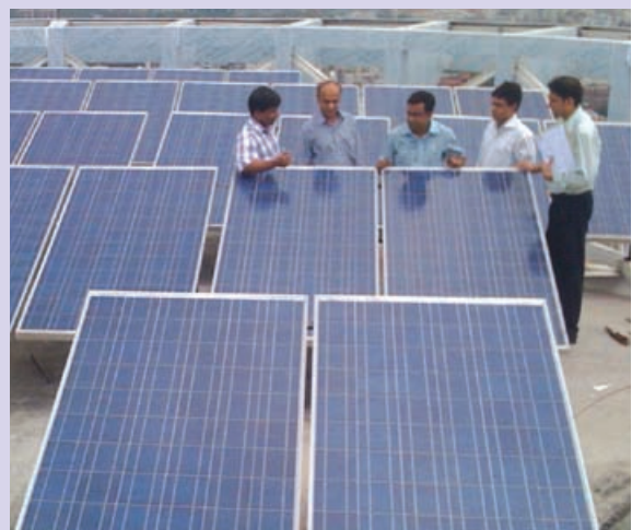
Inspection of Solar Panel in the consumer premises.
