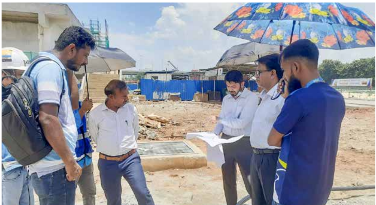
Inspection of Development Works by ED(Engineering) Engr. Jagodish Chandra Mandol at DESCO Uttara Area
