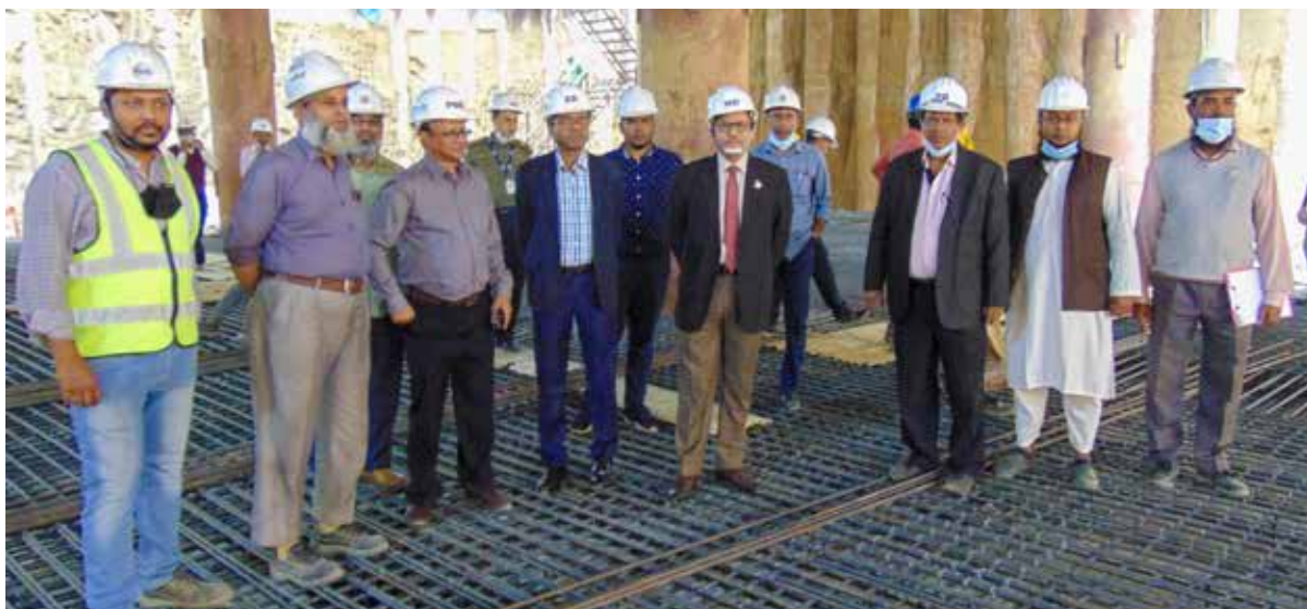
DESCO High officials lead by Managing Director inspected DESCO under construction 12 storied (with 06 Basement) Head Office building at Nikunja -2
