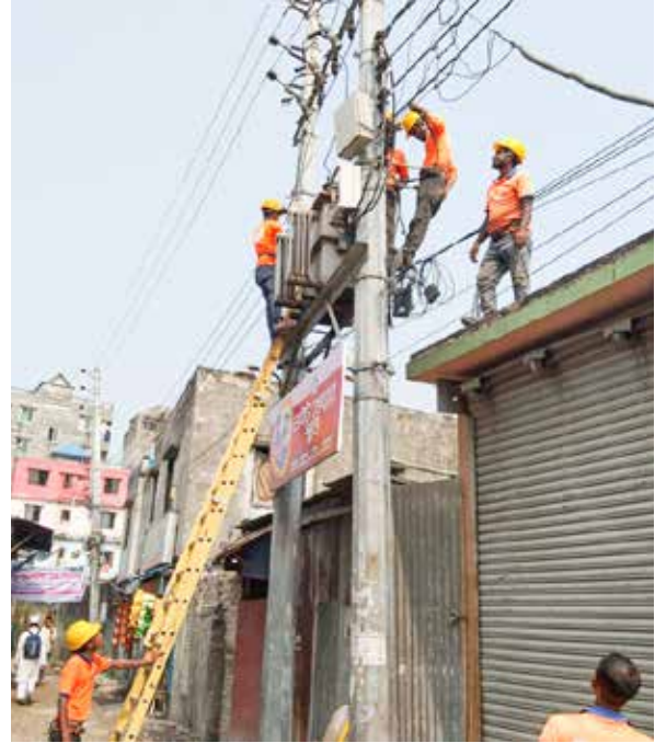
Damaged Transformer Changing Works of DESCO at Shahjadpur Area
