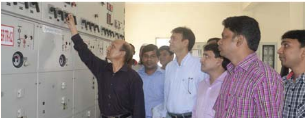
Energization of 33KV Source Line at Agargaon New 33/11 KV Sub-station
